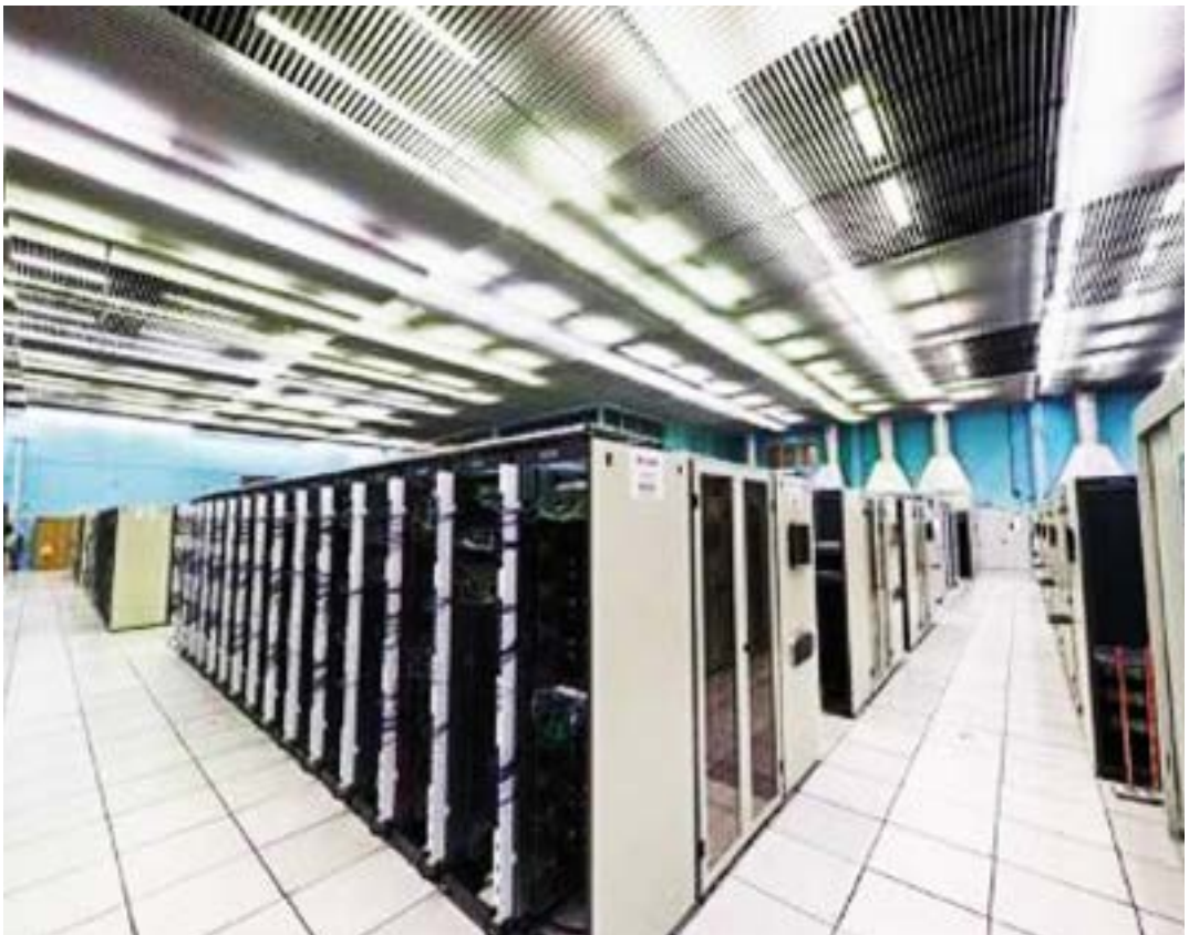
Servers, Storage and Data Centre Collocation Facility
