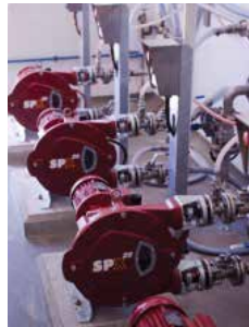
CHEMICAL DOSING ROOM
